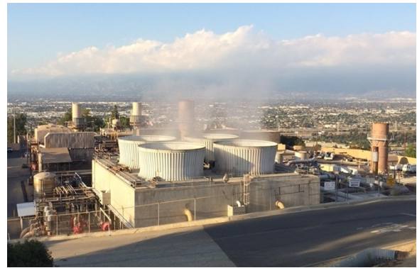
Figure 51. Puente Hills Landfill Gas Plant
