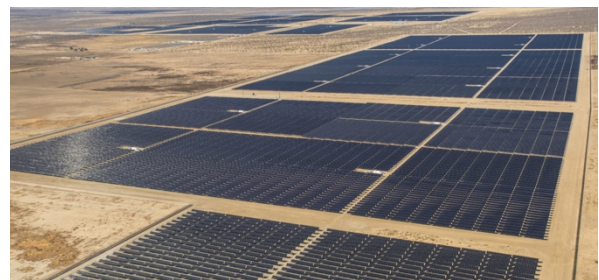
Figure 52. Astoria II Solar Photovoltaic Facility
