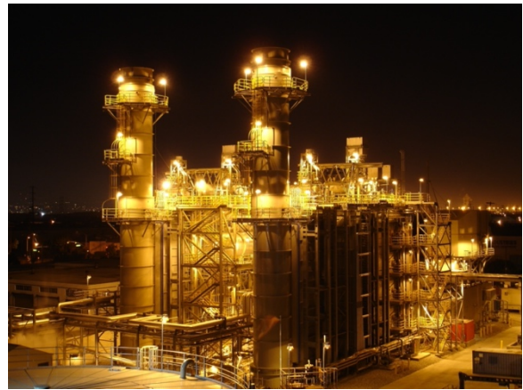
Figure 47. Malburg Generating Station
