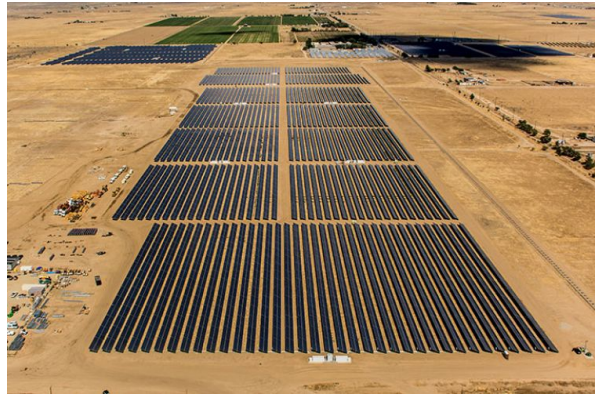
Figure 53. Antelope DSR 1 Solar PV Facility
