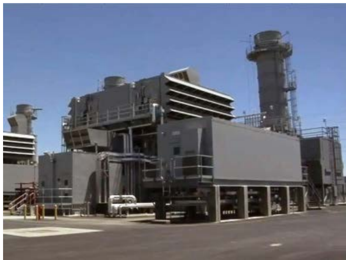
Figure 10. Almond II Power Plant
