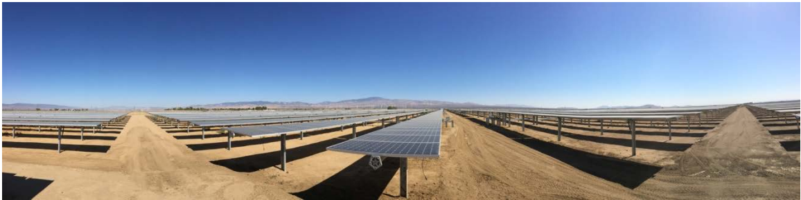
Figure 15. Rosamond West Solar 2 Facility
