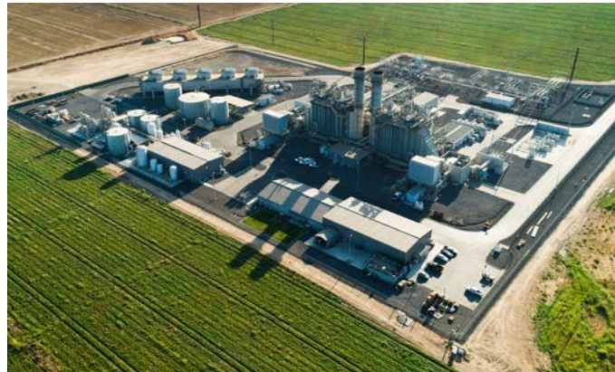
Figure 12. Walnut Energy Center
